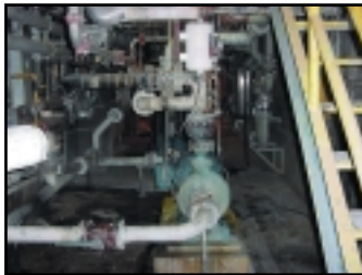
Sodium Silicate Load Out Pump. Goulds 3196MT Pump with AESSEAL® CDSA™ Double Mechanical Cartridge Seal and SSE10™ Barrier Fluid Tank System.
